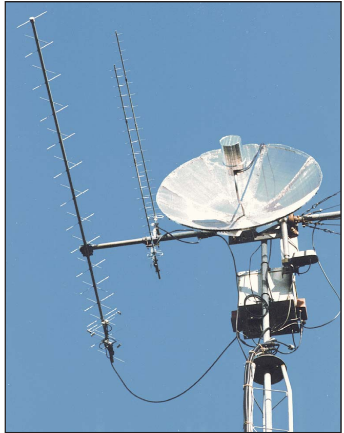
Fig 23.66—The completed and tower-mounted antenna system ready to go! The 40-W, 23-cm amplifier is enclosed in the box below the dish antenna.
