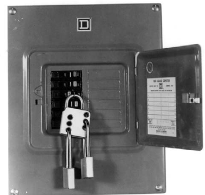
Fig 3.2 — If the switch box feeding power to your shack is equipped with a lock-out hole, use it. With a lock through the hole on the box, the power cannot be accidentally turned back on. (Photo courtesy of American ED-CO)
